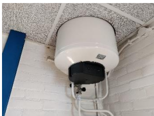
Figuur 3: close-up boiler
