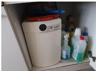
Figuur 4: close-in boiler
